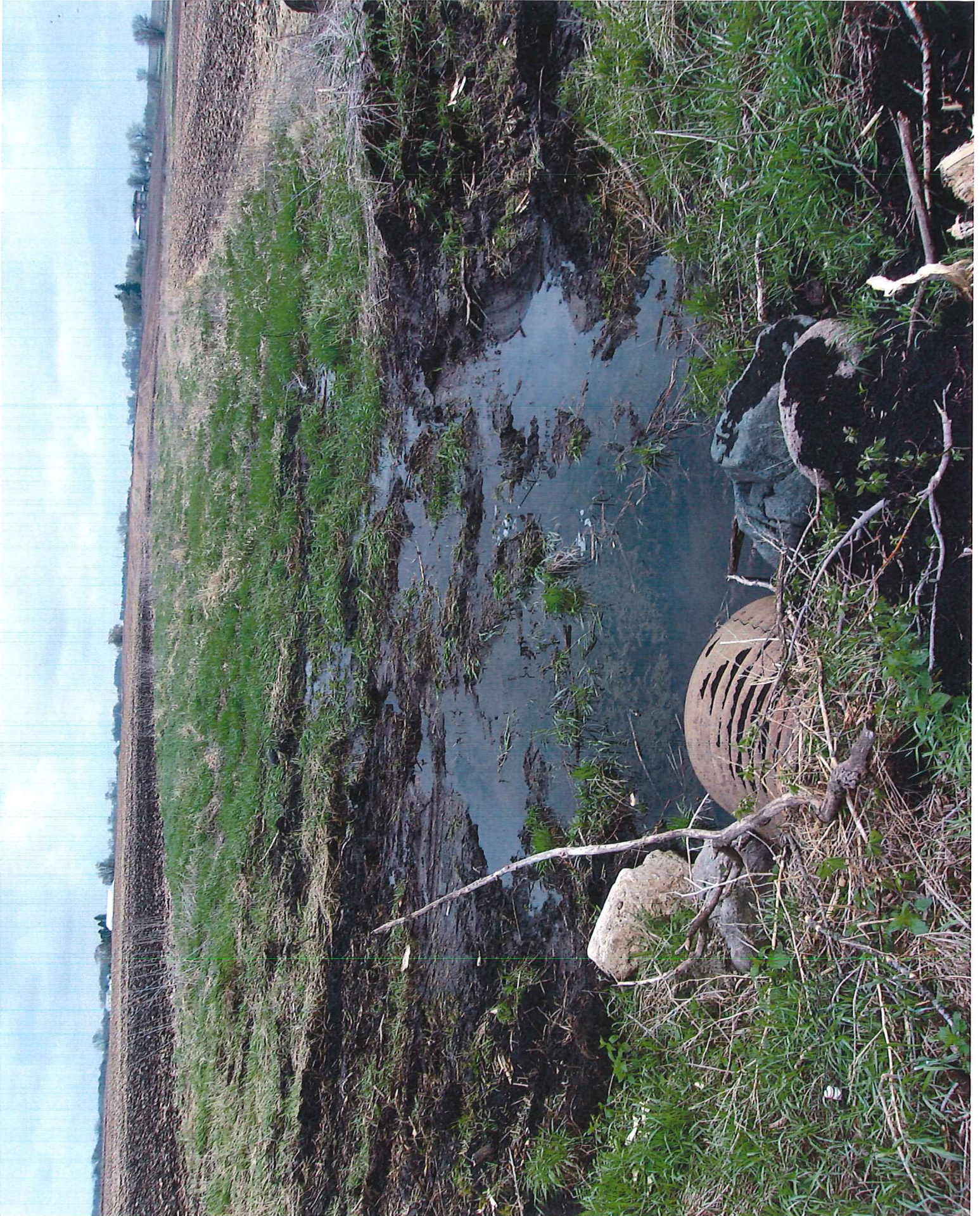
TILE WATER FLOWING ABOVE GROUND @ LAT 4 AREA ON MAIN
