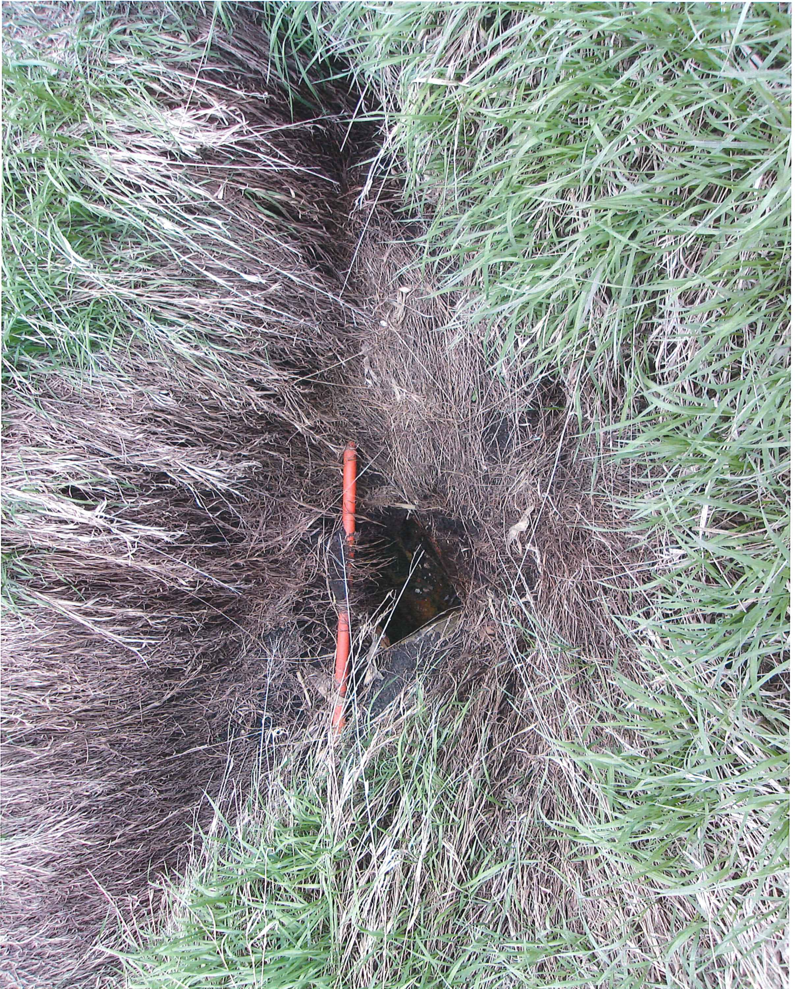
FIBER OPTIC CABLE IN TILE
